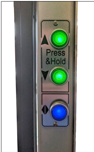
Upper level control panel Call station incorporated in to upper level gate post.
