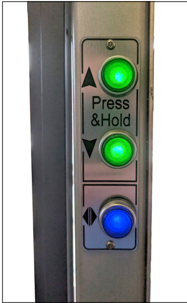
Upper level control panel Call station incorporated in to upper level gate post.
