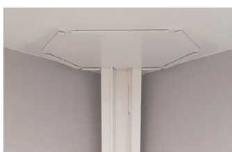
Fire seals for both levels
